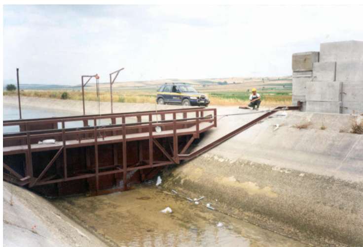
Installation of the steel frame to deviate the water to the by-pass canal
