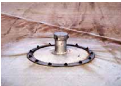
Aeration and evacuation of gas
