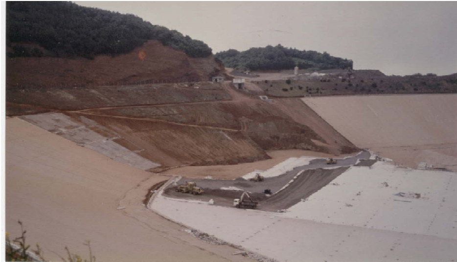
Project of Barlovento: 1st drainage layer of 8/40 Separation layer geotextile 500 g/m 2 - 2nd drainage layer of 0/6
